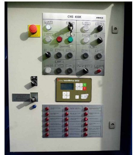
Pic. 5: View behind the protection door on the control cabinet
